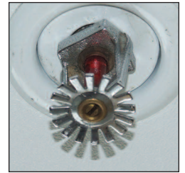
Sprinklers reduce the risk of home fire death by 83%.
